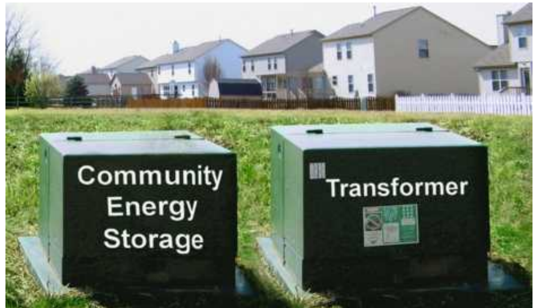
20 Li-Ion community energy storage units on Detroit Edison grid
