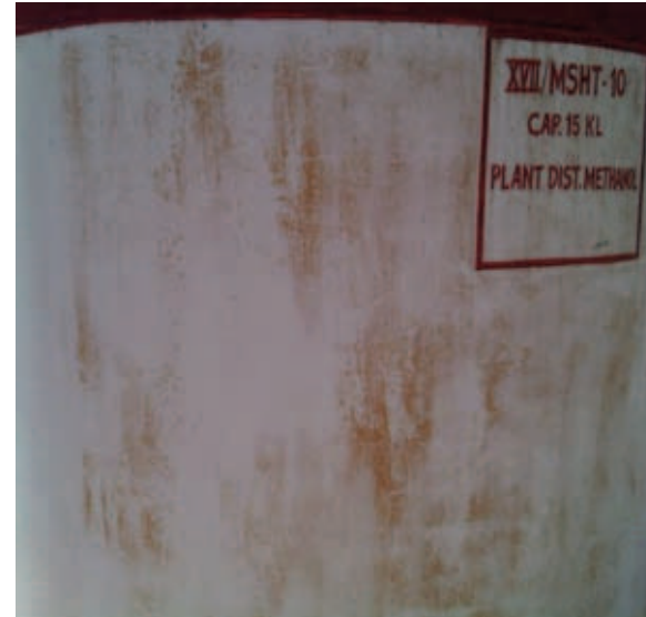
Before Coating- Corroded MS Tank
