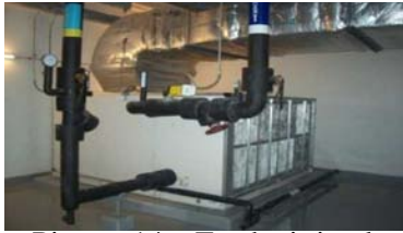
Picture 14 – Fresh air intake
