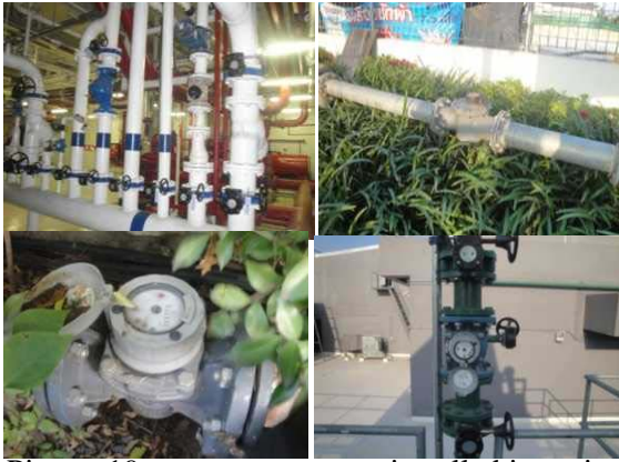
Picture 19 - water meters are installed in various places ,e.g main section pipe, cooling tower
