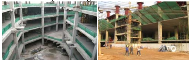
Picture 41- Use of green mesh to prevent fall of material and dust pollution
