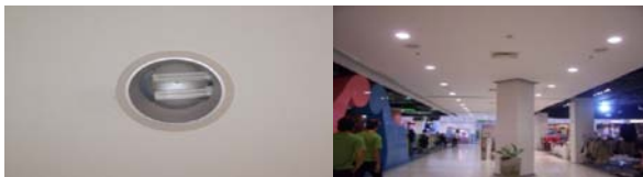
Picture 10 - Compact fluorescent lamp downlight with high luminaire efficiency and controlled with electronic ballast
