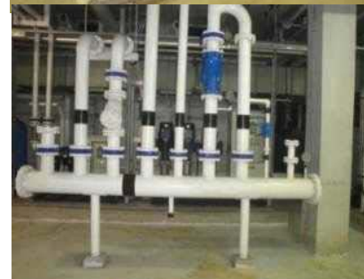
Picture 22 - the waste water recycling system
