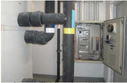
Picture 9 –VSD control the AHU motors
