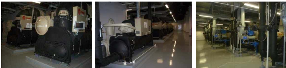
Picture 5 – High Efficiency Chiller plant
