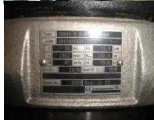
Picture 18 - High Efficiency Motor
