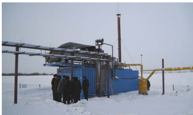
Fig. 1. Genset station in a container mode
