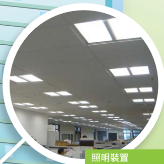
照明裝置 Lighting installation
