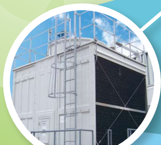
空調裝置 Air-conditioning installation
