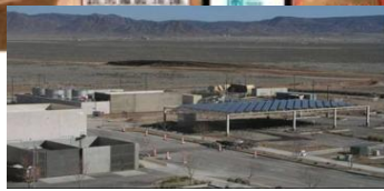
Dispersed power, energy storage equipment and PV system
